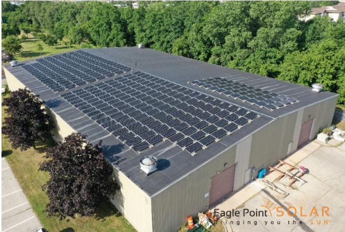
Municipal Service Center: 100 kW
