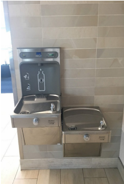
Figure 13: Water bottle filling station and drinking fountain on second floor
