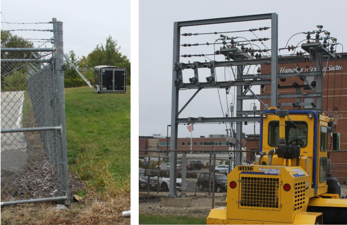
Electrical Transformer at the Edge of the Site.
