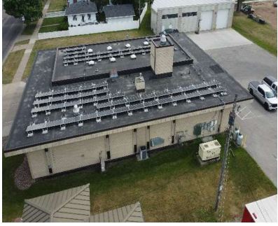
Fire Station #3: 30 kW
