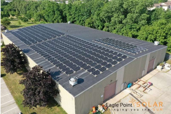
Municipal Service Center: 100 kW
