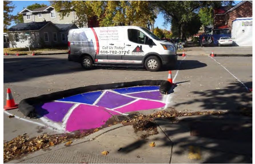
Figure A-10: A temporary curb extension at Jackson Street and 8 th Street
