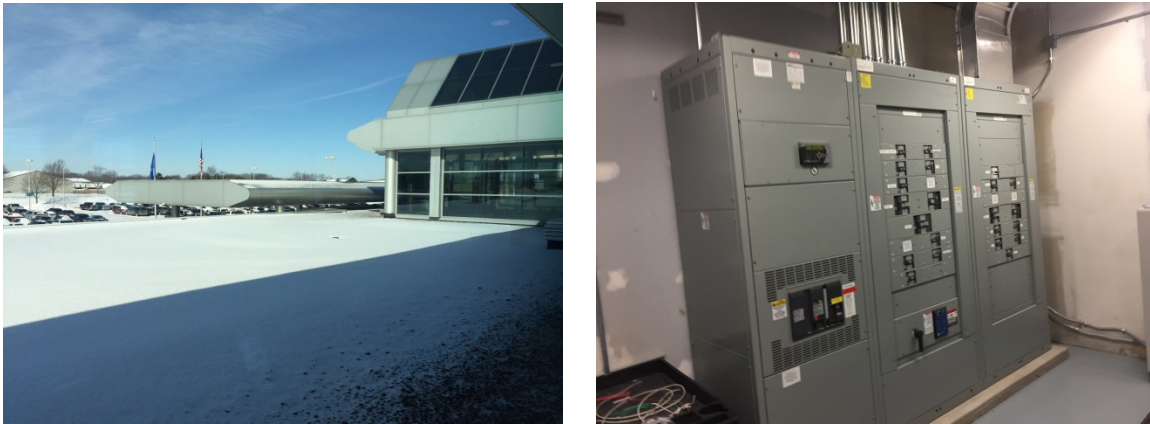
Figure 1- Terminal rooftop view (typical) and incoming electrical service panel
