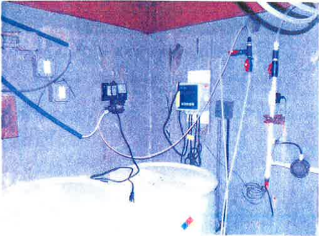
Acid Barrels in Work Area
