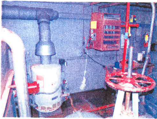
Water Heater is Replaced Every 2 Years Due to Harsh Environment
