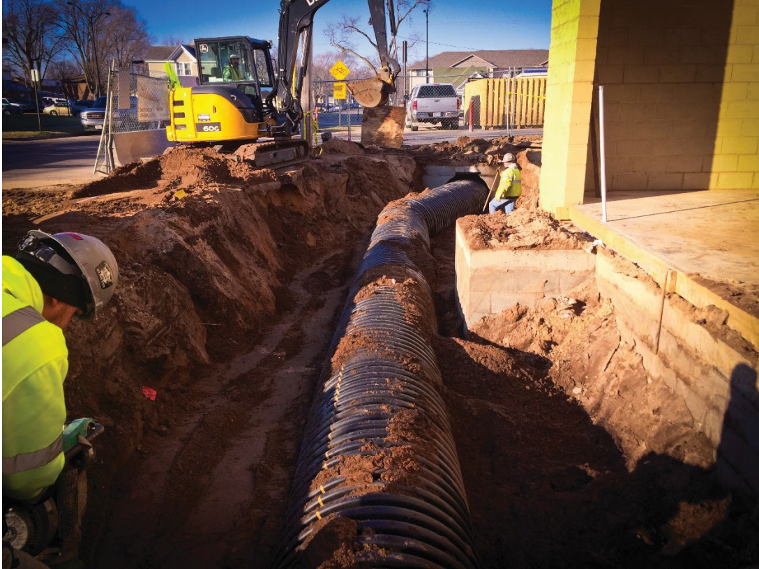
Underground Stormwater Management System 507 N 13 St La Crosse, WI - AGUILERA
