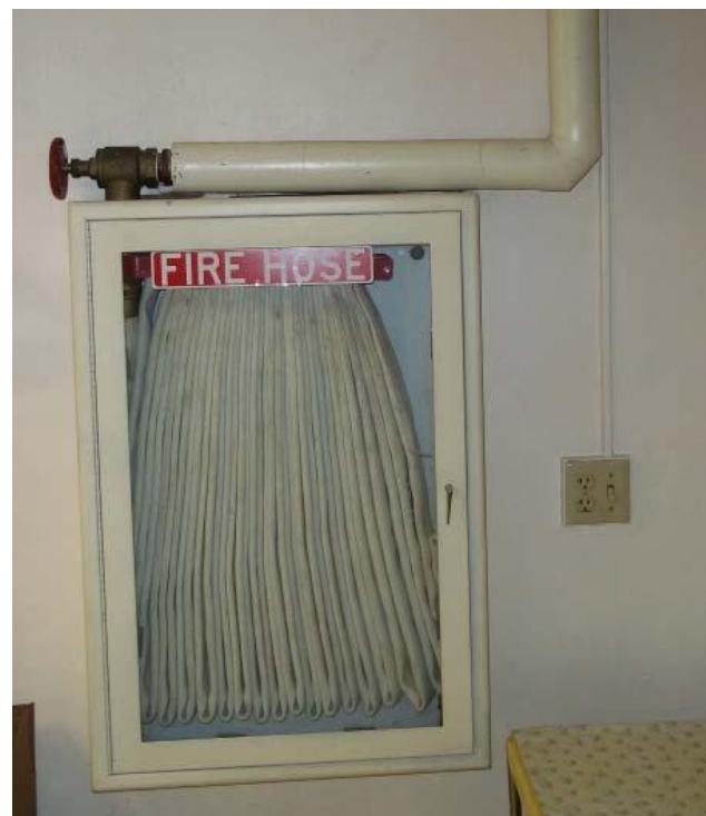
Lower level fire hose. (2012)
