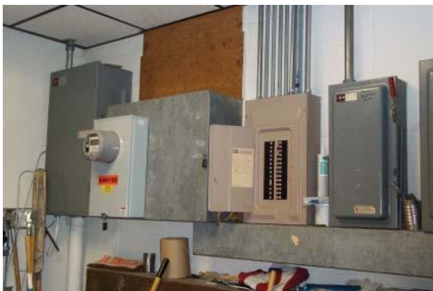
Multiple metering cabinets, load centers, and switches. (2012)
