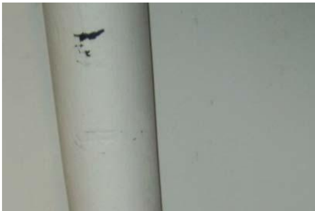
Fire hose water supply pipe. (2012)
