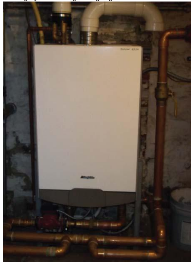
New boiler installed in 2010. (2012)
