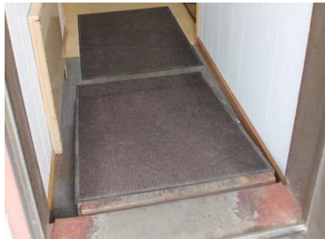
"Temporary" ramp at rear exit. (2012)
