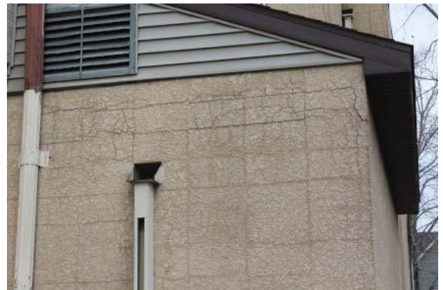
Cracked EFIS walls of 1977 addition. (2012)
