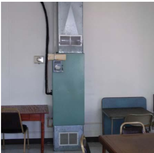
Cooling system vertical fan-coil. (2012)
