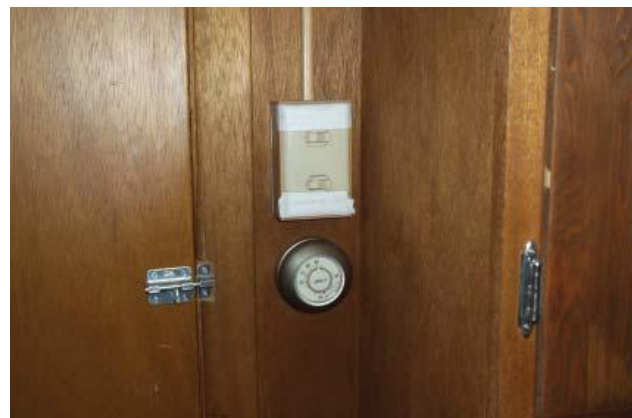
Typical light switches. (2012)
