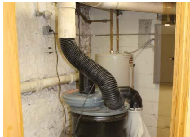
Mechanical room located under central egress stair. (2012)
