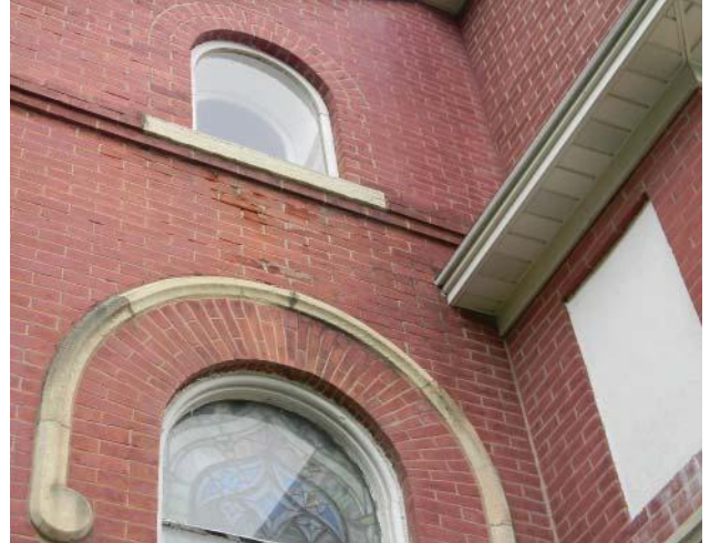
South wall of original building showing masonry deterioration.
