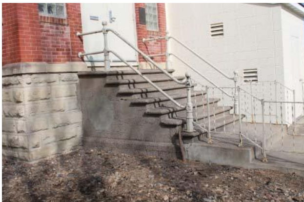
Brick and Foundation condition at south elevation (2012)
