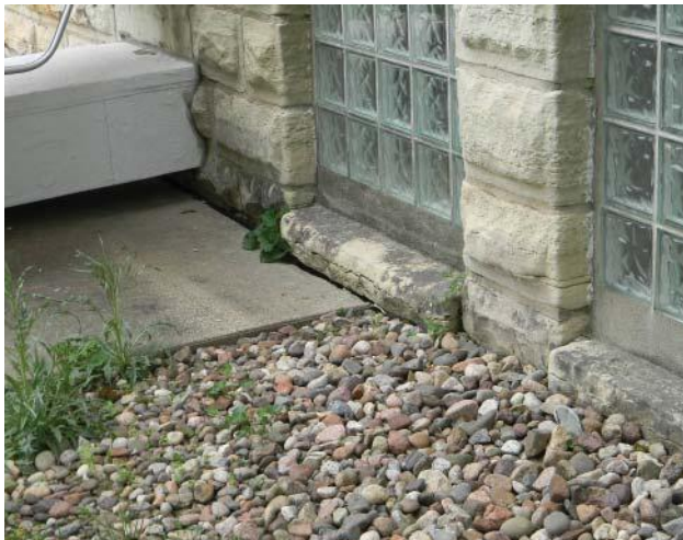
West wall of original building showing limestone deterioration.
