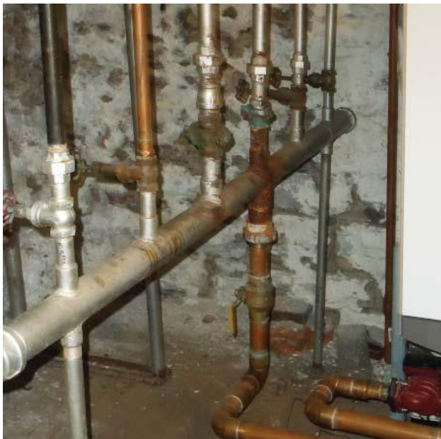
Older piping and valves for heating system. (2012)
