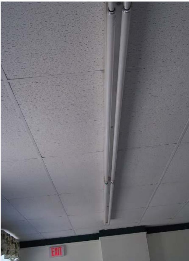
Typical fluorescent strip lighting. (2012)
