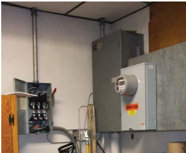
Multiple metering cabinets, load centers, and switches. (2012)
