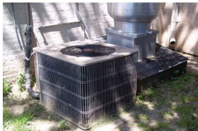
Exterior compressor-condensing unit at grade. (2012)
