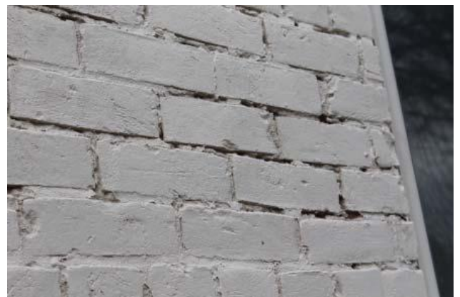
Typical painted brick condition. (2012)
