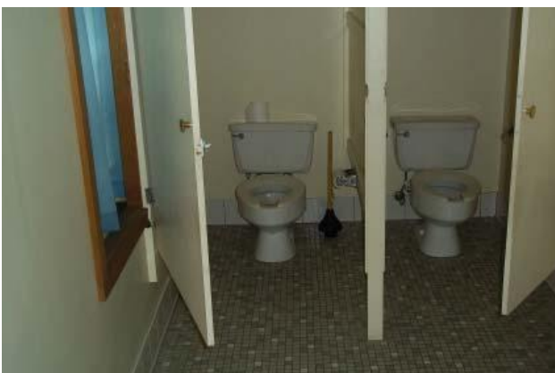
Toilet fixtures in second floor women's restroom. (2012)
