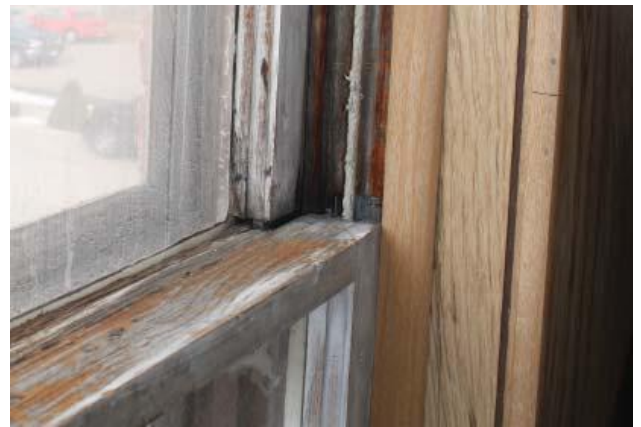
Typical window condition on second floor. (2012)
