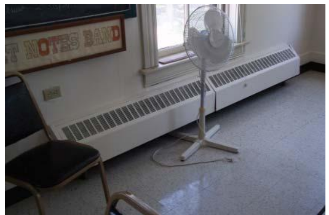
Finned tube radiation heating equipment. (2012)
