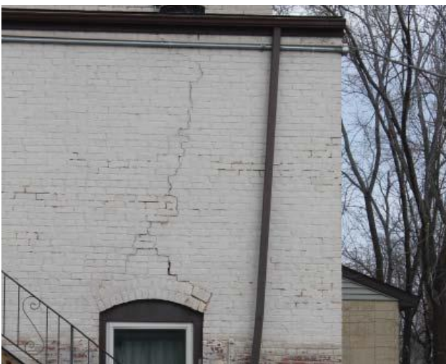
Condition of brick above south east window. (2012)
