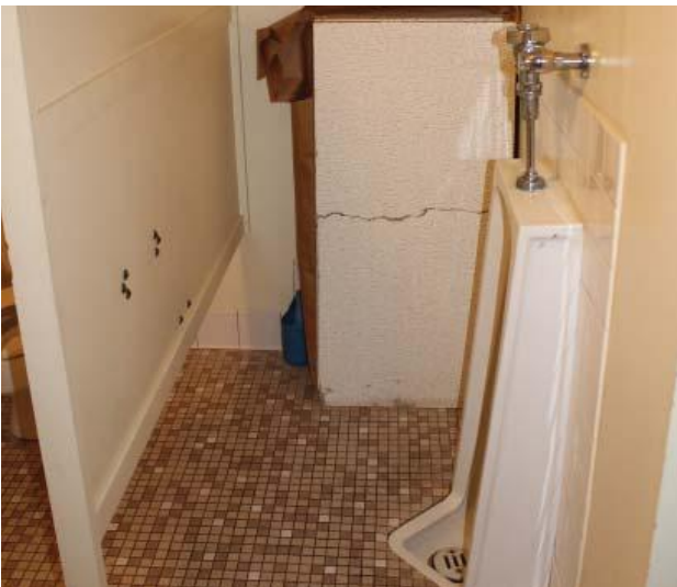
Men's room used for building material storage. (2012)
