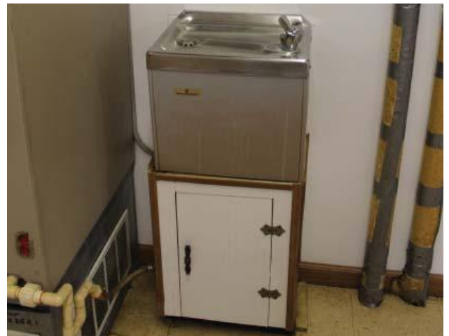
Inaccessible drinking fountain. (2012)
