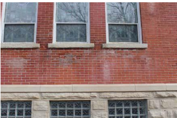
Sill and window condition at west elevation (2012)
