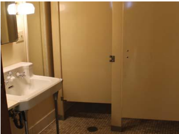
Out-dated and inaccessible first floor restrooms. (2012)
