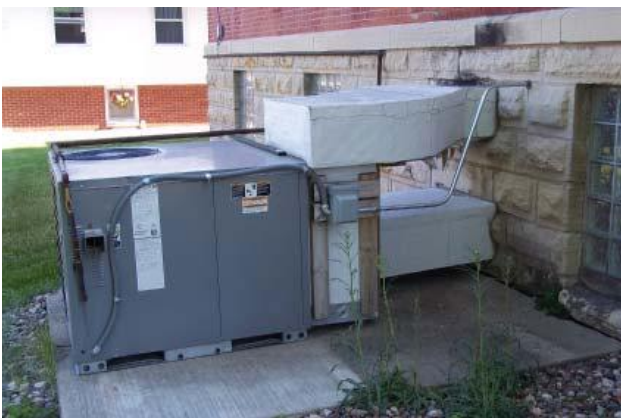
Rooftop heating unit located at west side on grade. (2012)
