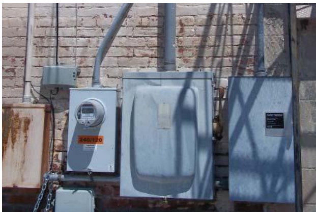
Exterior electric service switching. (2012)
