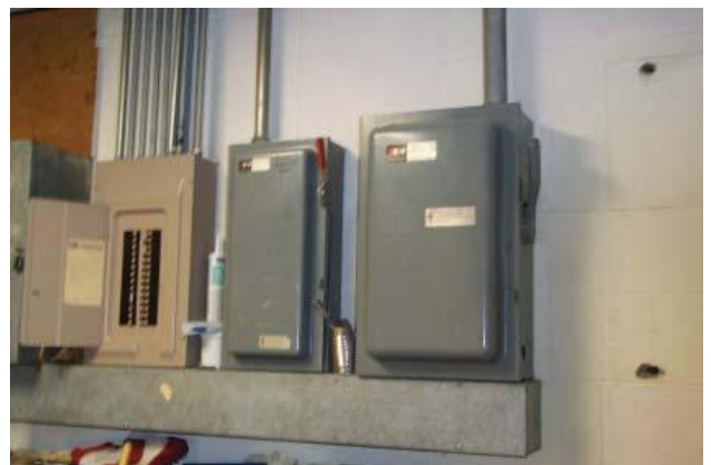
Multiple metering cabinets, load centers, and switches. (2012)
