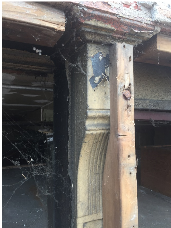
Figure 32 – Original cast iron storefront column. July 2017.
