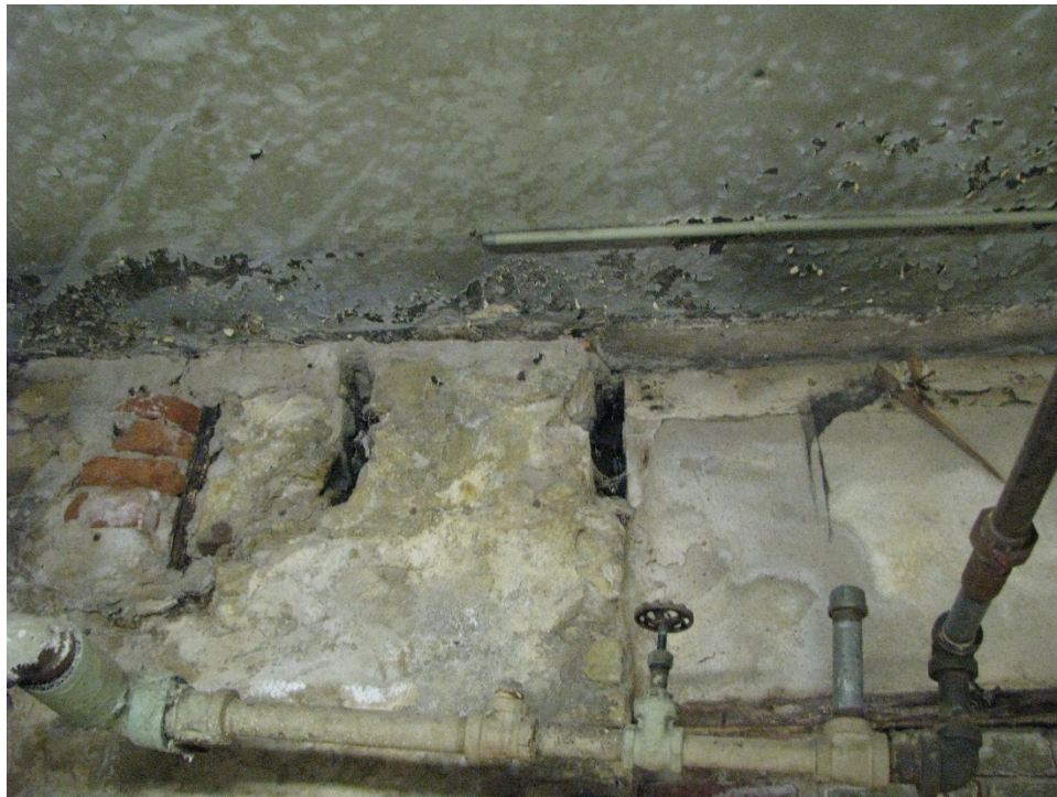
Figure 18 – Remnants of old wood floor joists below current concrete floor slab. January 2017.
