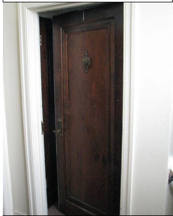
Figure 26 – Apartment entry door. January 2017.
