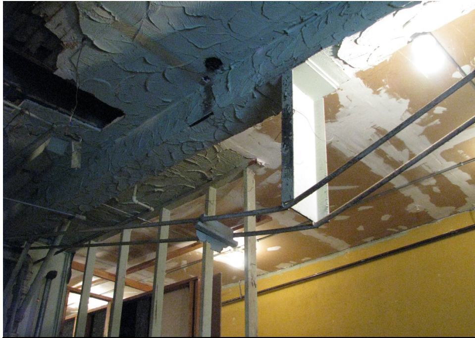
Figure 20 – Compromised structure (missing column) on first floor. January 2017.
