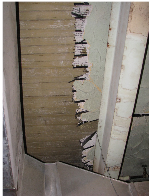
Figure 22 – Remnants of beadboard ceiling, first floor. January 2017.
