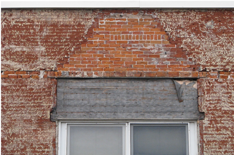
Figure 30 – Detail of bay window remnants. September 2017.
