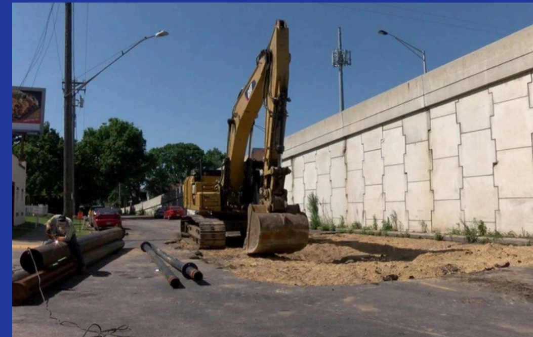
Sinkhole near Gould & Avon, 2013
