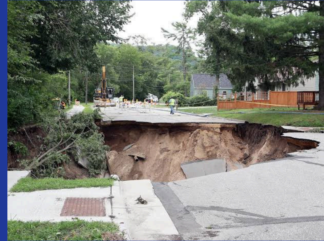
Sinkhole near Myrick Park along Marsh, 2017
