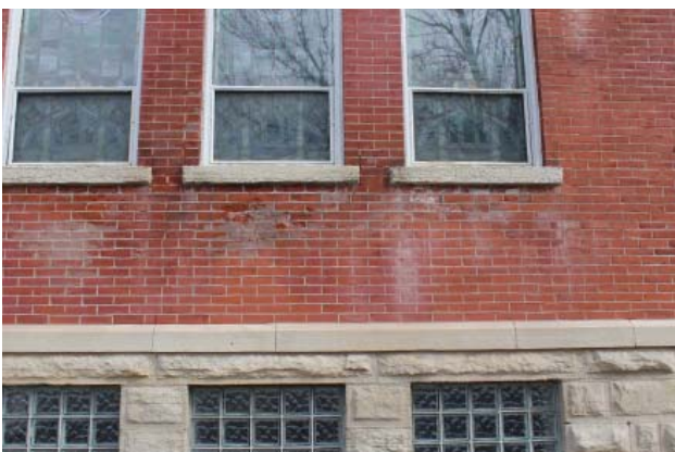
Sill and window condition at west elevation (2012)
