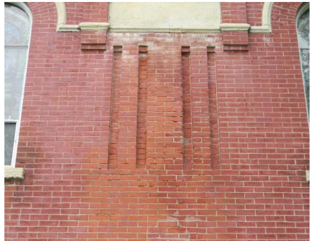
West wall of original building showing masonry deterioration.
