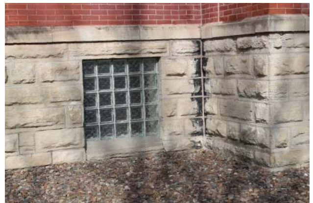
Foundation and Sill condition at south elevation (2012)
