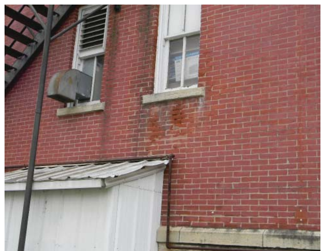
North wall of original building showing masonry deterioration.
