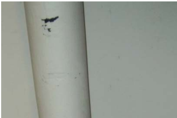
Fire hose water supply pipe. (2012)
