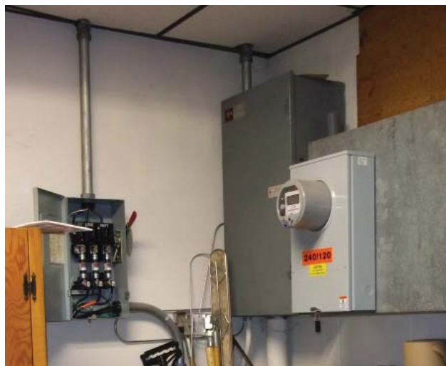
Multiple metering cabinets, load centers, and switches. (2012)
