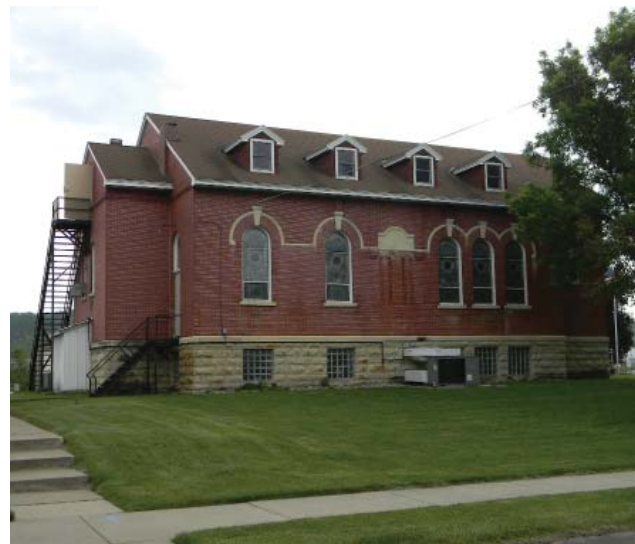
West wall of original building showing masonry and stone deterioration.
