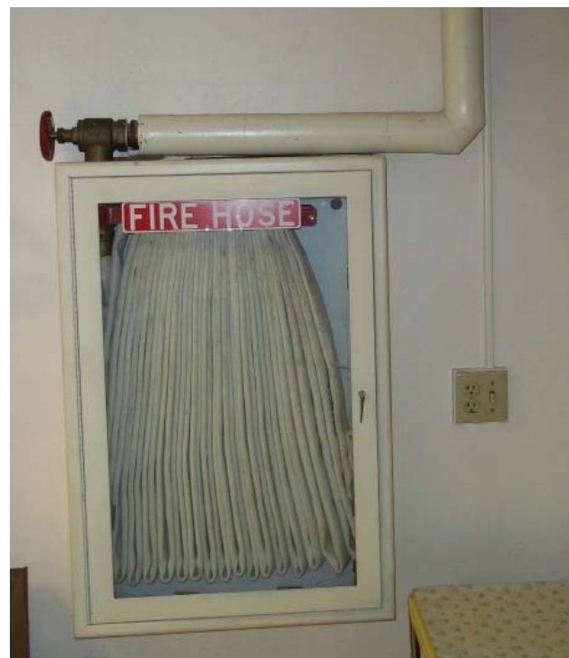
Lower level fire hose. (2012)
