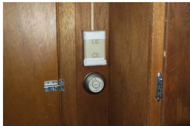
Typical light switches. (2012)
