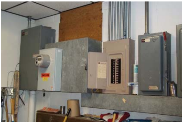
Multiple metering cabinets, load centers, and switches. (2012)
