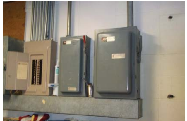
Multiple metering cabinets, load centers, and switches. (2012)
