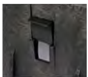
Temporary drop port
