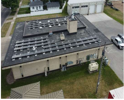
Fire Station #3: 30 kW
