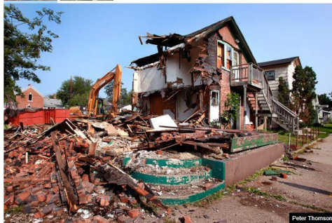
A demolition crew makes progress on razing a condemned five-plex rental at 1524 10th St. S. Peter Thomson
