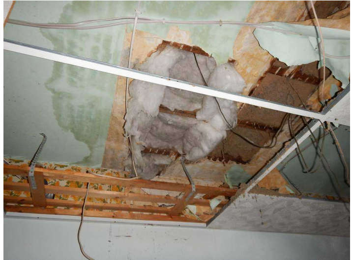
Ceiling Family Room Prior Moisture
