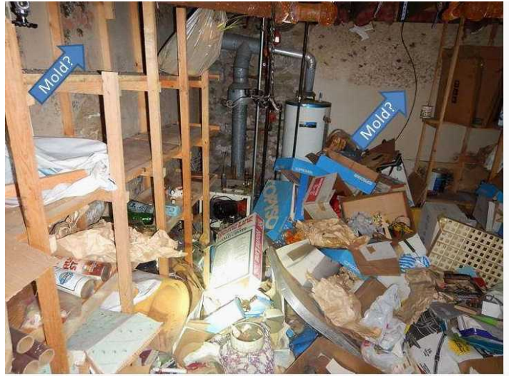
Basement Possible Mold
