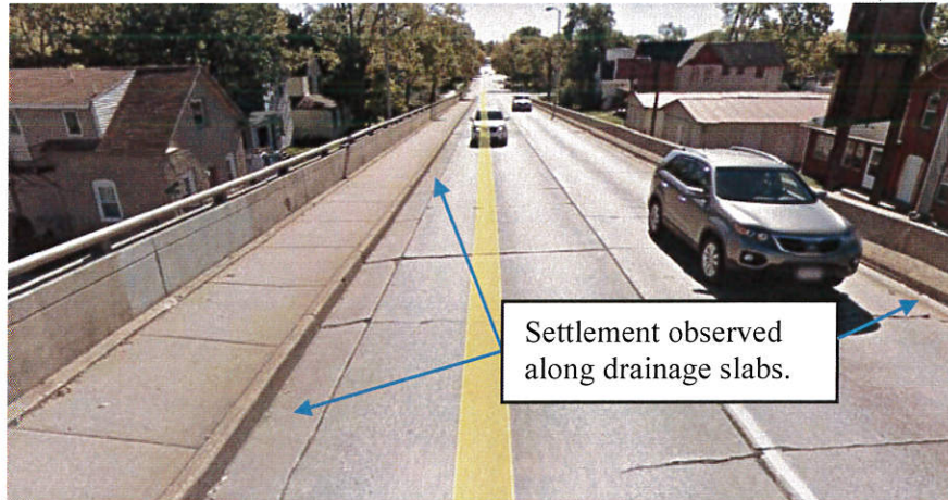
Figure 7 - Rose St. bridge showing the deck surface to be scanned and settlement issue.
