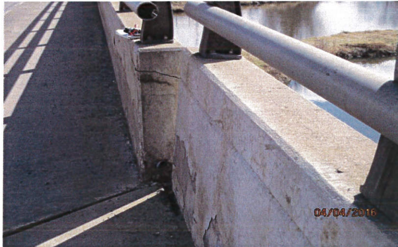
Figure 6 – Evidence of Settlement of Lang Drive Bridge
