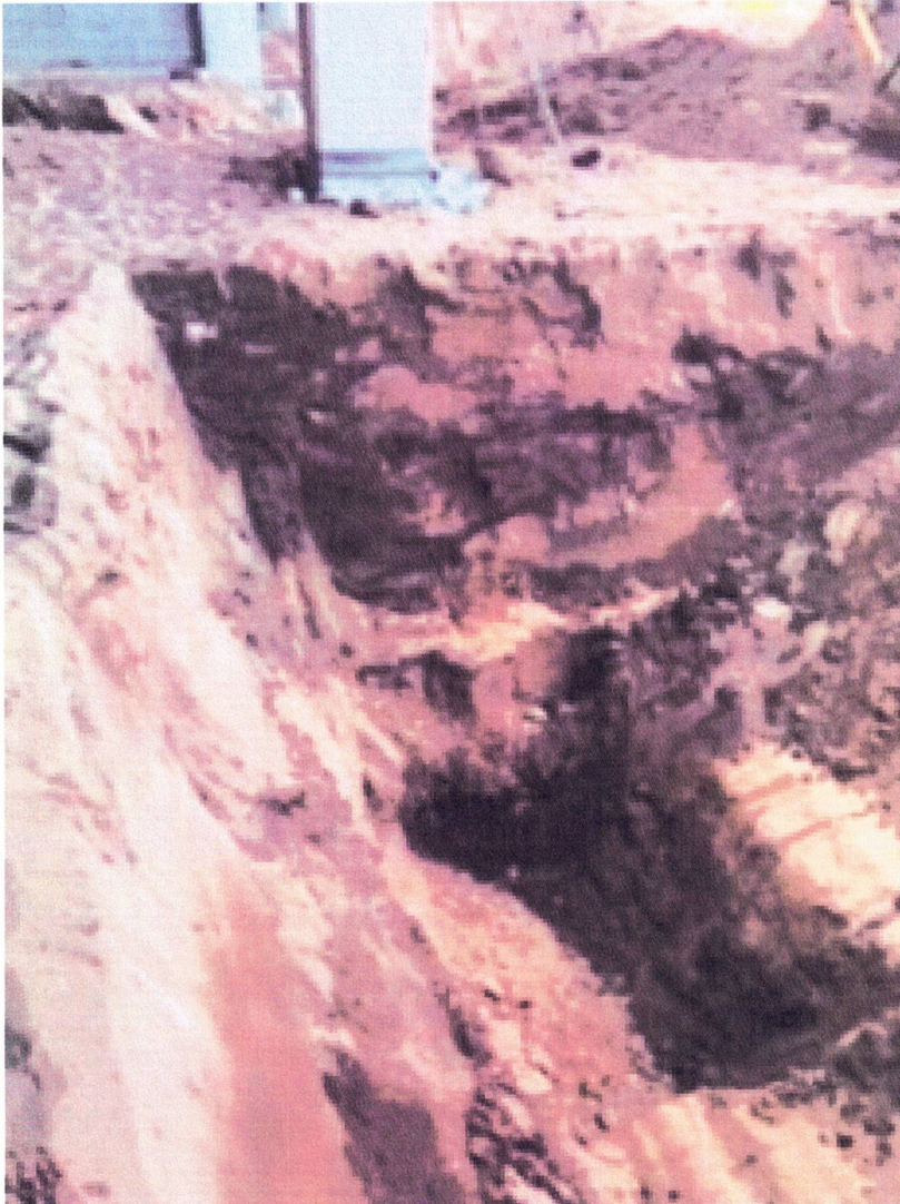
Debris found in excavation at 11/R
