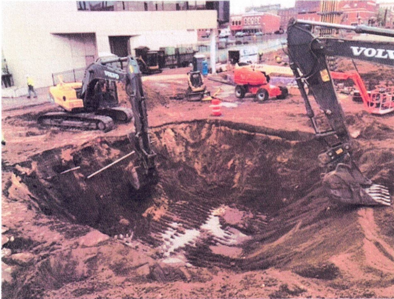
Bottom of 6' over dug excavation for column at gridlines 2.3/D measures approximately 24'x24'
