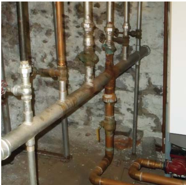
Older piping and valves for heating system. (2012)
