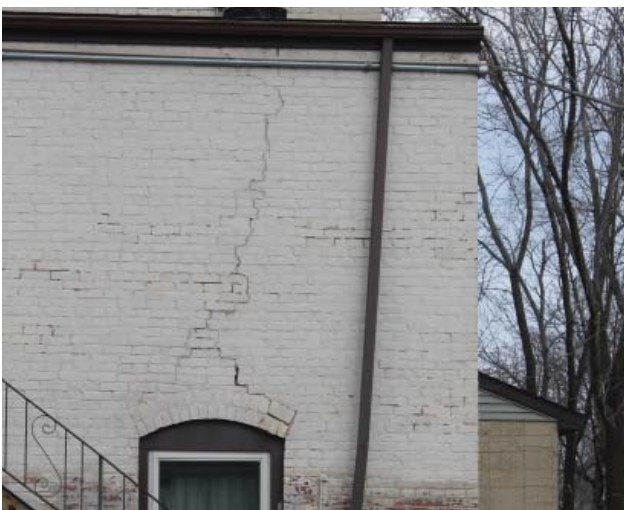
Condition of brick above south east window. (2012)
