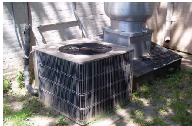
Exterior compressor-condensing unit at grade. (2012)
