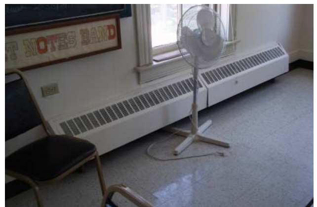
Finned tube radiation heating equipment. (2012)
