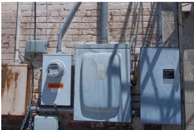
Exterior electric service switching. (2012)
