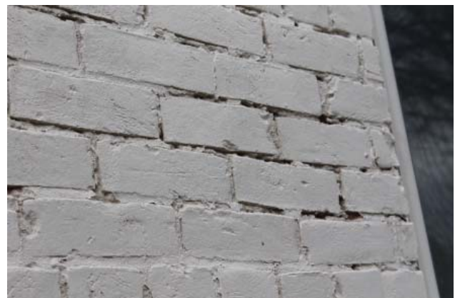
Typical painted brick condition. (2012)
