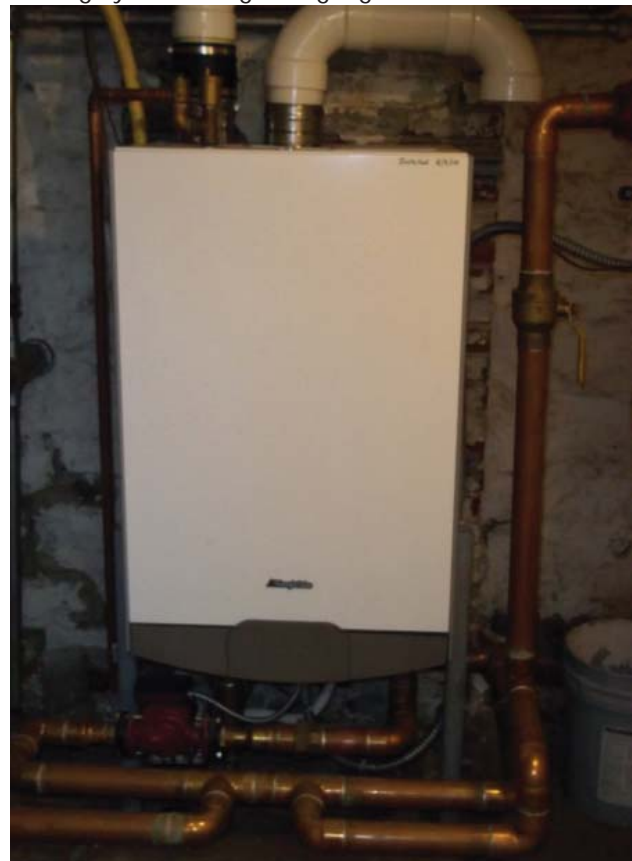
New boiler installed in 2010. (2012)
