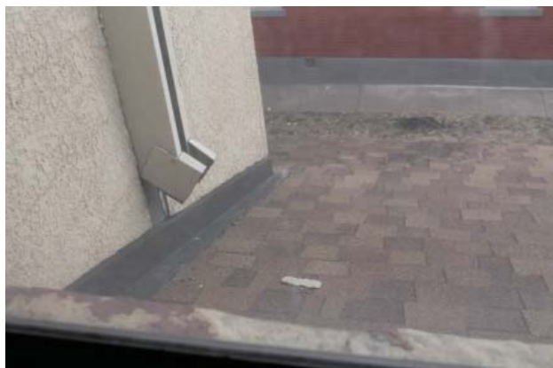
Roof over storage addition (damaged sill in foreground). (2012)
