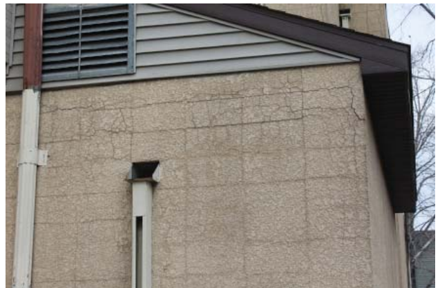
Cracked EFIS walls of 1977 addition. (2012)
