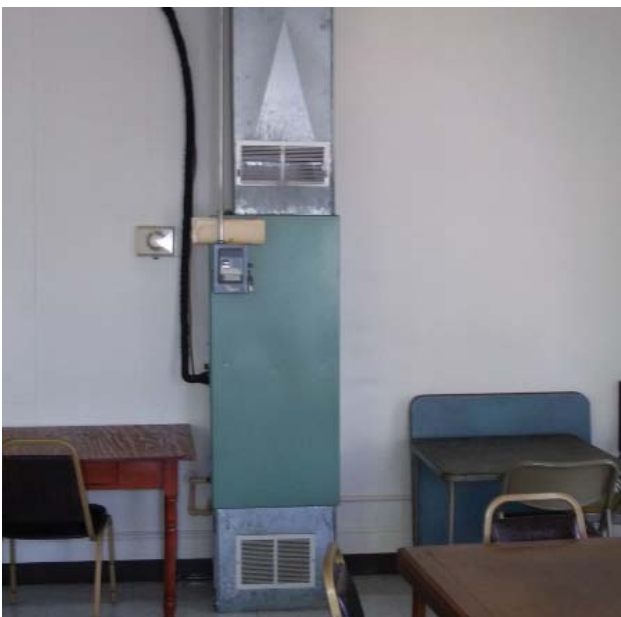
Cooling system vertical fan-coil. (2012)
