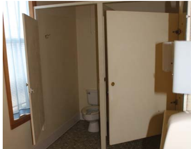
Partition obscuring restroom window. (2012)
