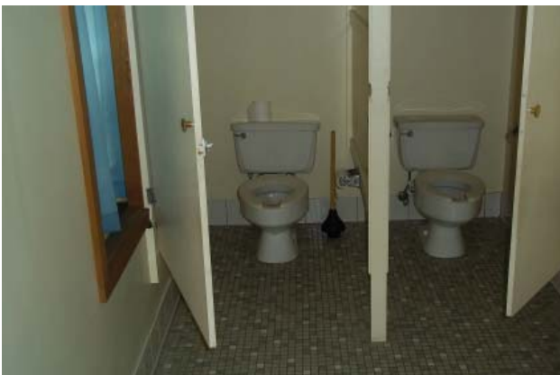
Toilet fixtures in second floor women's restroom. (2012)
