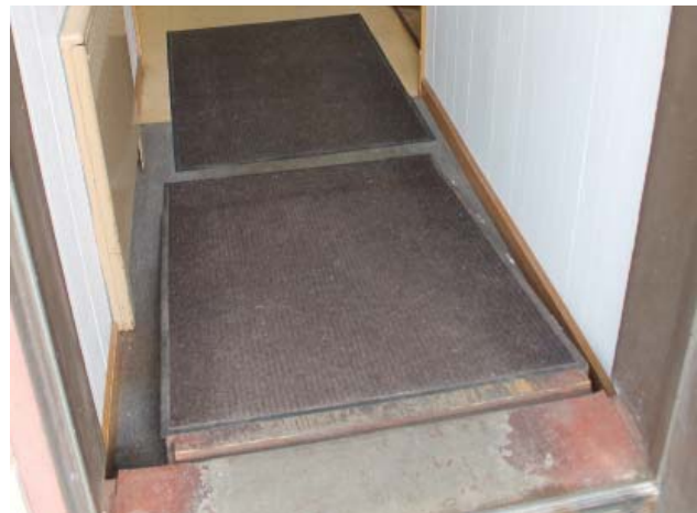
"Temporary" ramp at rear exit. (2012)
