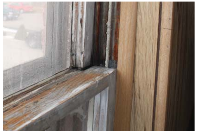
Typical window condition on second floor. (2012)
