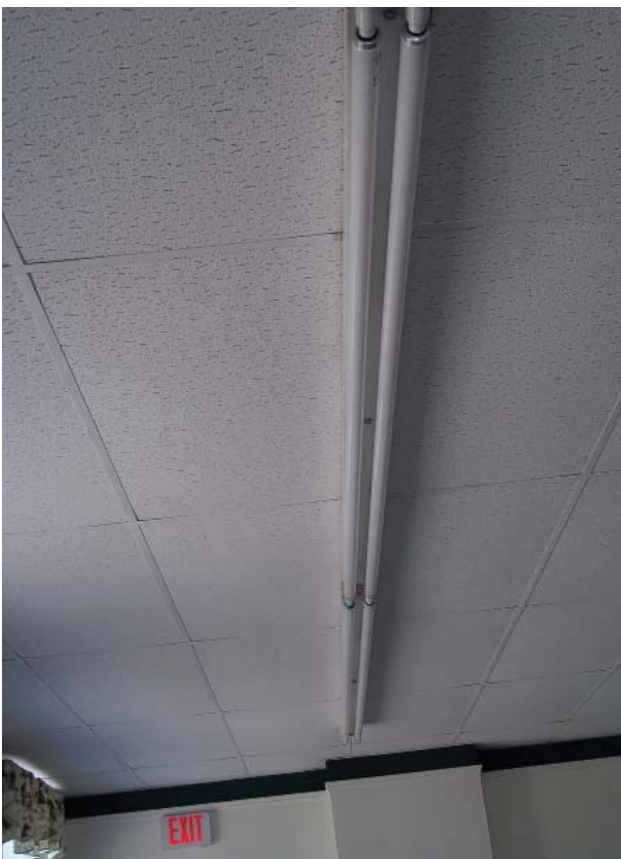
Typical fluorescent strip lighting. (2012)
