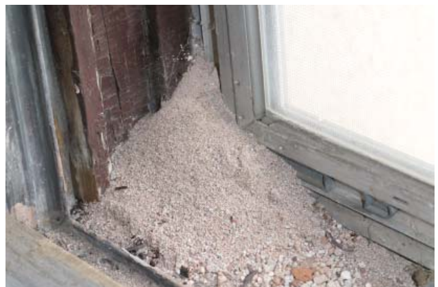
Brick debris at interior of second story window. (2012)
