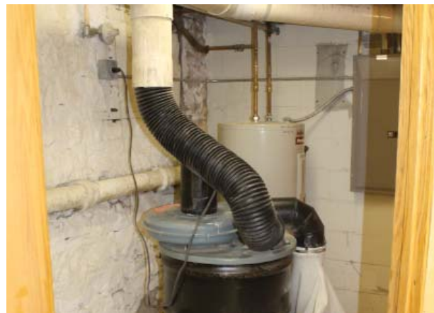
Mechanical room located under central egress stair. (2012)
