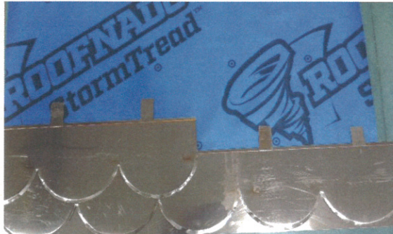
Band Shell Roof Assembly: the 16 gage copper fish-scales sheets are cleat-together in rows which are then fastened through the ice-sheild onto the plywood decking with copper clips and nails.
