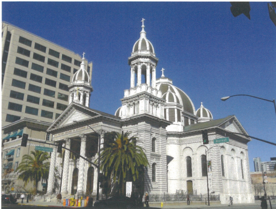
Replacing a tin roof, Gundersen detailed the cathedral's new copper and composite roof.
