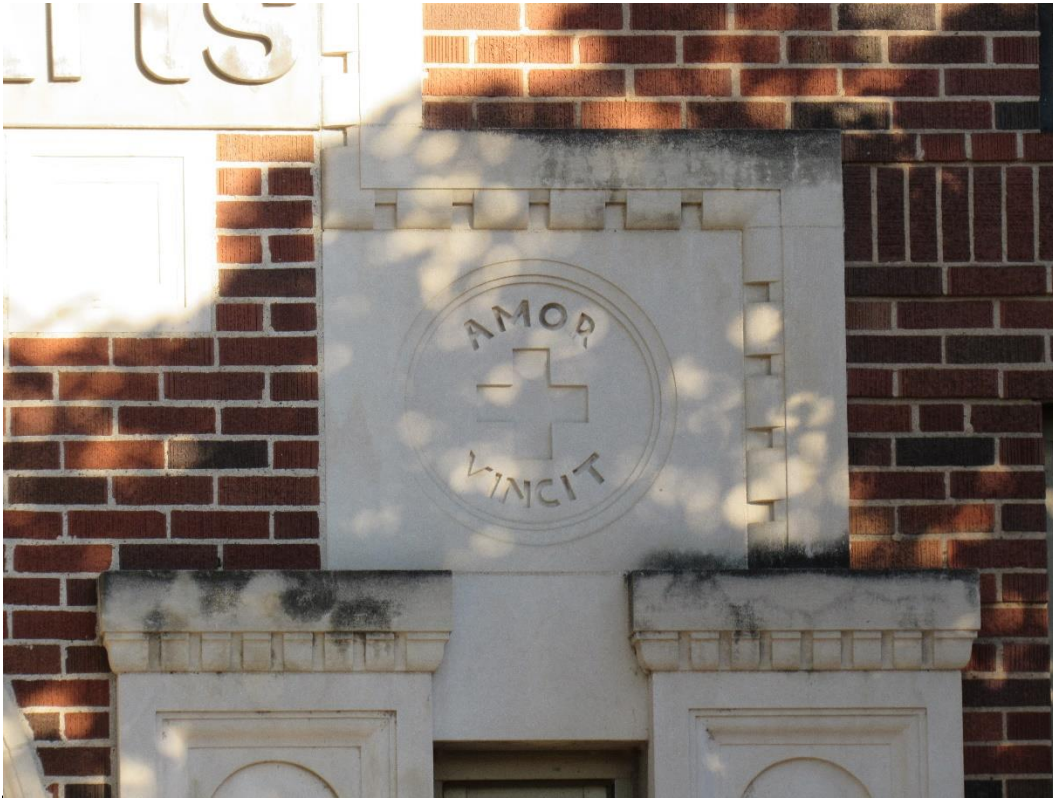
Figure 15 – Detailed view of the carved limestone at School of Nursing Entry. October 2025.
