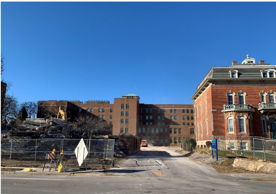
Figure 18 – View of the west façade at the School of Nursing. During the St. Ann’s demolition. November 2025.
