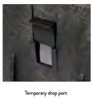
Temporary drop port
