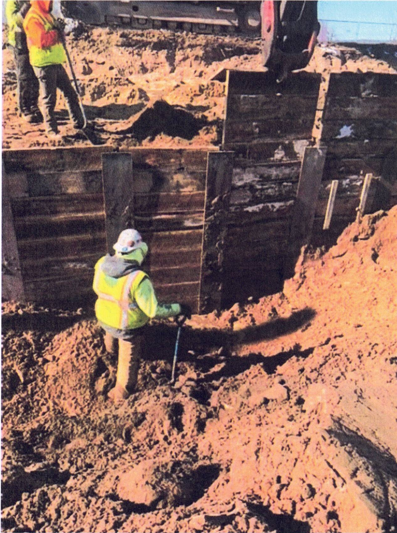
Excavation observation showing groundwater and shoring for columns at gridlines 2.3/B & 10/B.
