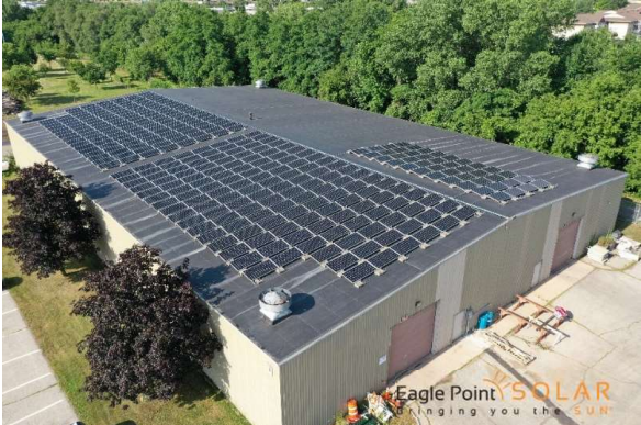
Municipal Service Center: 100 kW
