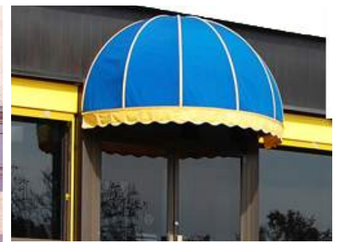
Example of Unacceptable Awning
