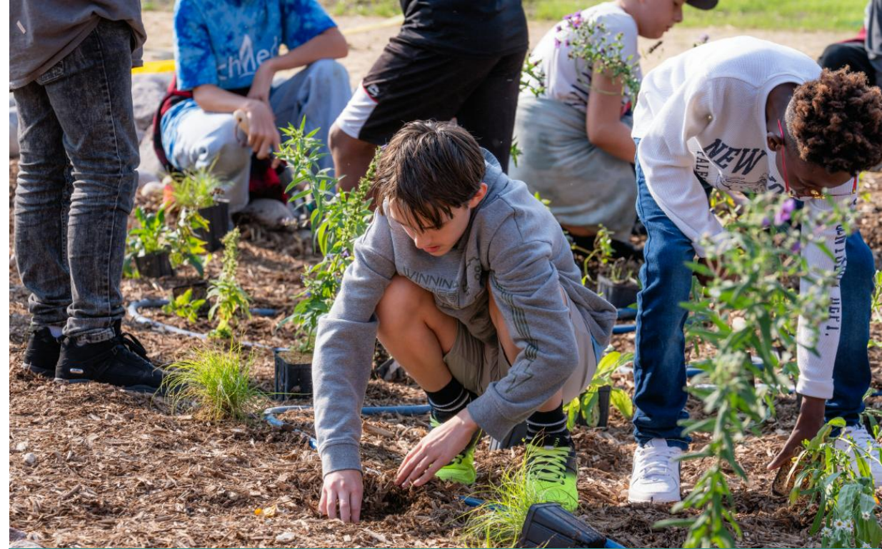
La Crosse students install a rain garden at their school to help mitigate stormwater runoff
