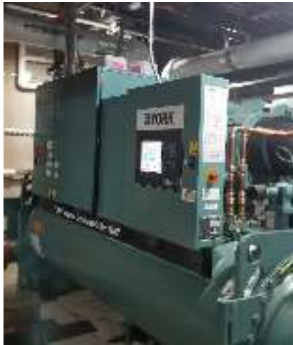
New York Chiller
