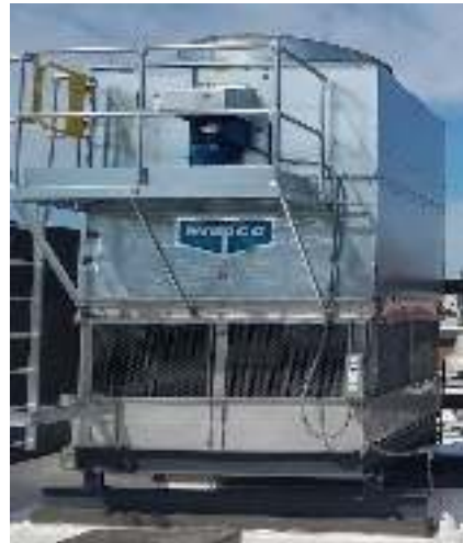
New Cooling Tower
