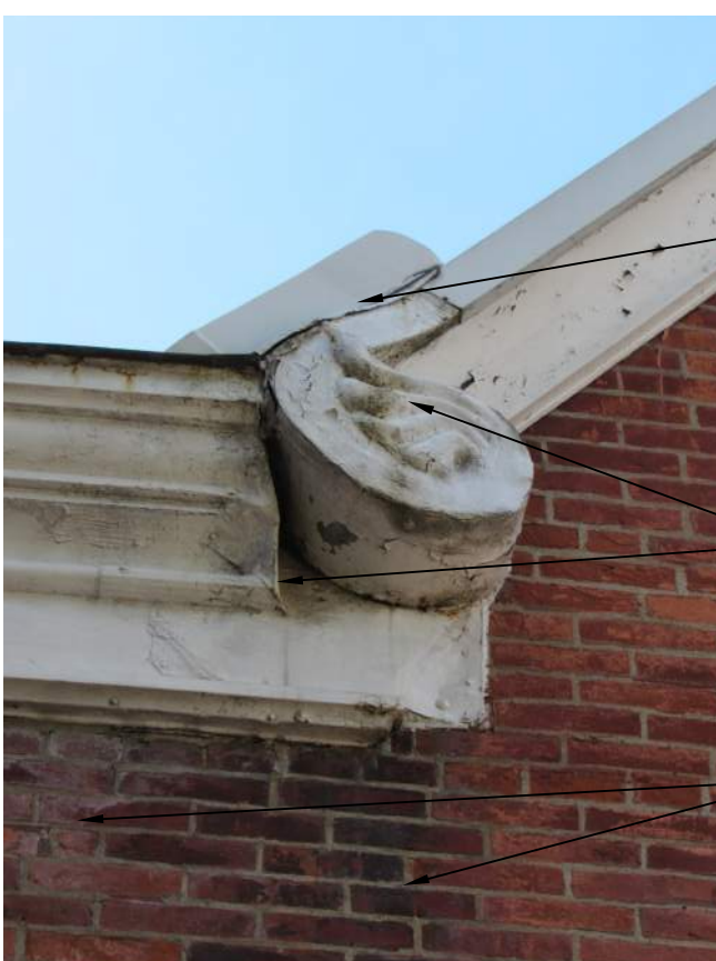
P6 CORNICE DETERIORATION NO SCALE
