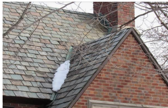
Figure 26 – The ridge on the dormer is damaged, possibly letting in water (2026).
