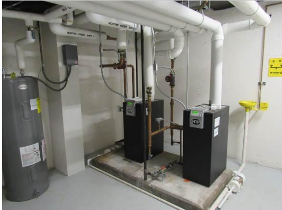
Figure 106 – The mini-boilers were installed circa 2020 (2026).
