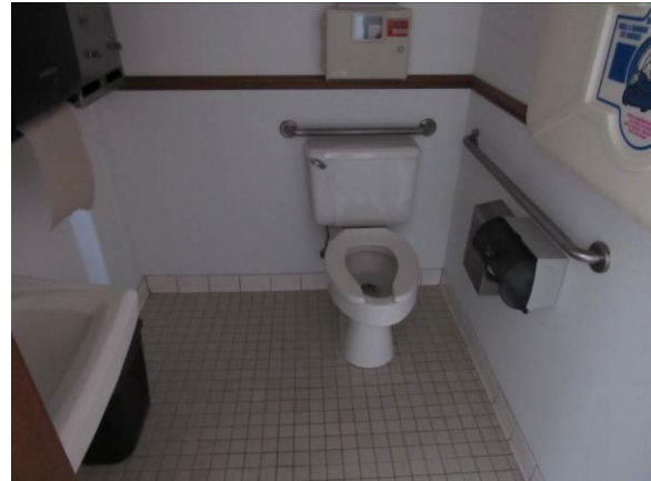
Figure 41 – The restrooms do not appear to be large enough to comply with current ADA requirements (2026).
