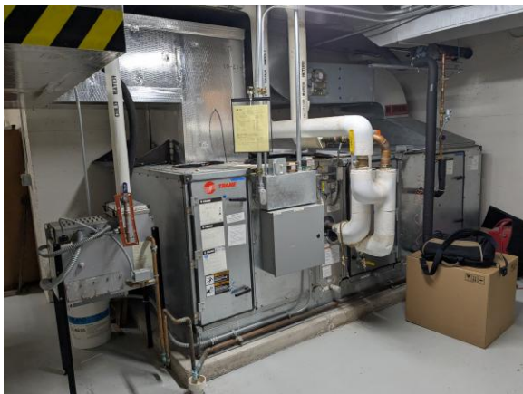
Figure 61 – New Air Handling Unit in Basement (2026).
