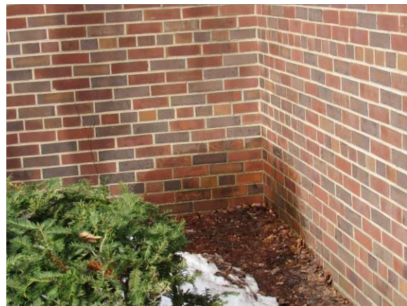
Figure 11 – Water runs off the roof, splashes at grade and saturates the walls (2026).
