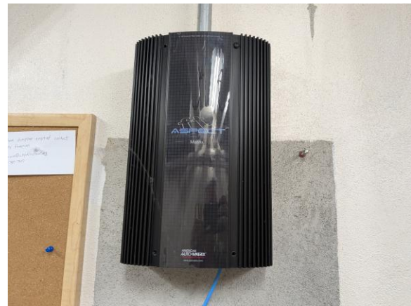
Figure 64 – Energy Management System installed at this Facility (2026).
