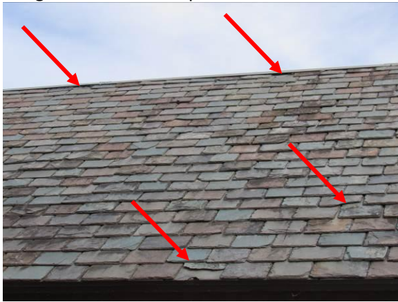
Figure 113 – There are some damaged slate shingles on the roof (2026).
