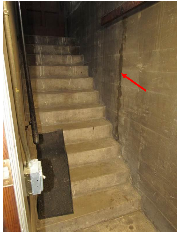
Figure 51 – The stairs at the south end of the basement, notice the water (2026).
