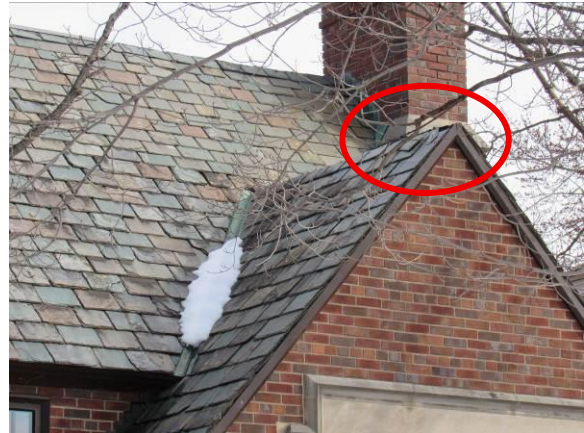
Figure 53 – The broken ridge slate and missing metal cap may be contributing to the roof leak (2026).
