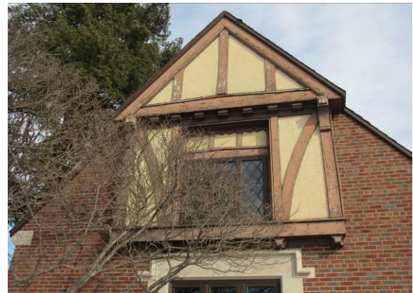
Figure 14 – Peeling paint and rusted nails are evident on the trim at the gable (2026).
