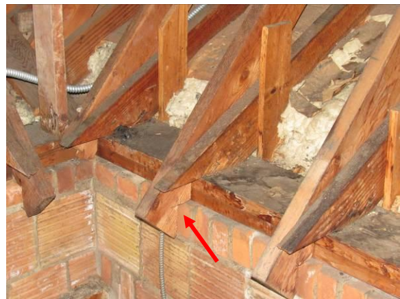
Figure 59 – Rafter ends were cut with a bird's mouth over the sill plates (2026).
