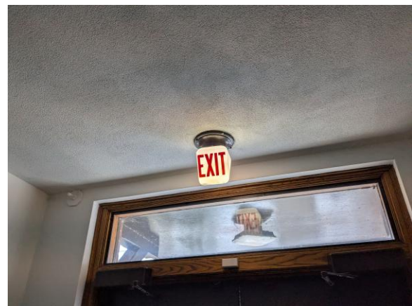
Figure 71 – Antiquated EXIT Light on the Main Level of the Library (2026).
