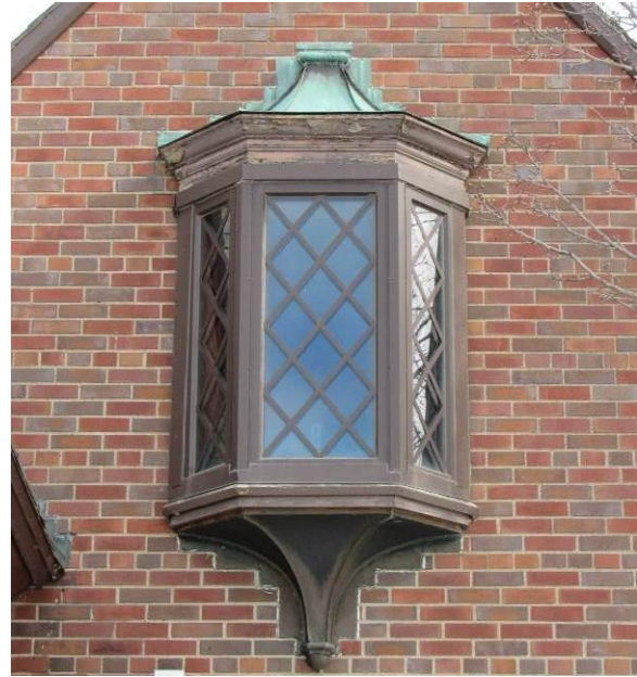
Figure 13 – Oriel window has peeling paint and modern replacement windows (2026).
