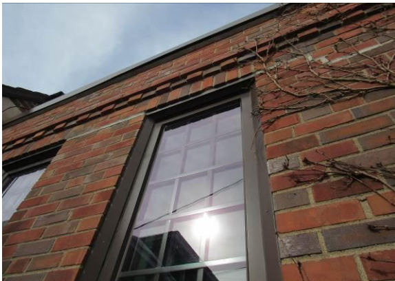
Figure 22 – Previous masonry repairs are evident at the window heads (2026).
