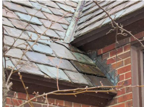
Figure 25 – Copper valley and step flashing is used to channel water off the roof (2026).
