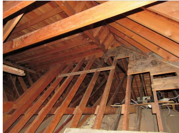
Figure 58 – Complex roof forms meet over the front entry with parallel gables and a cross gable, notice the cross bracing and collar ties (2026).
