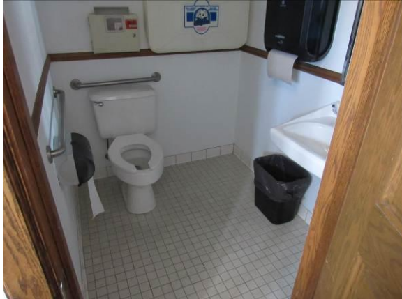
Figure 104 – The restrooms nearly comply with ADA requirements, but are still deficient in a few areas (2026).
