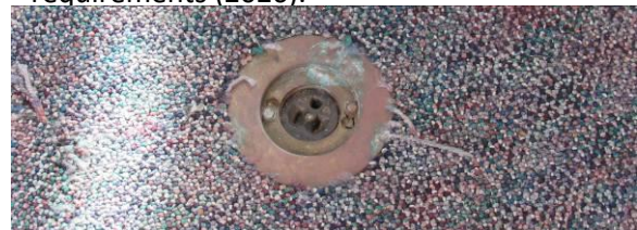
Figure 42 – Floor outlets may contain old wiring (2026).
