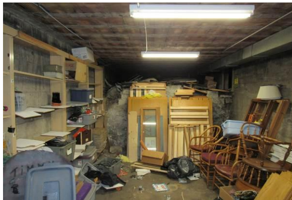
Figure 109 – Some older fluorescent fixtures remain in the basement (2026).
