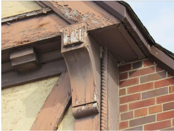
Figure 117 – The wood trim should be cleaned, primed, and painted the next time any exterior work is done to the walls or roof (2026).
