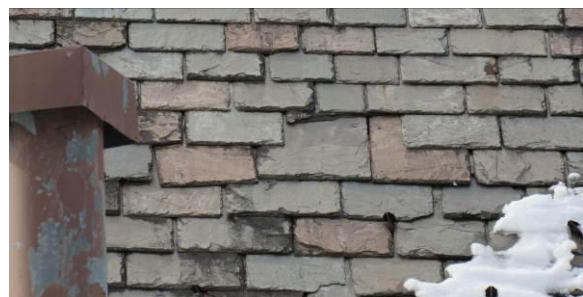
Figure 27 – Damaged and missing slate shingle should be replaced (2026).
