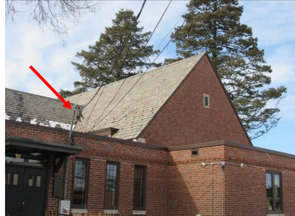
Figure 107 – Existing electrical service has seen better days, underground service would be a big upgrade (2026).
