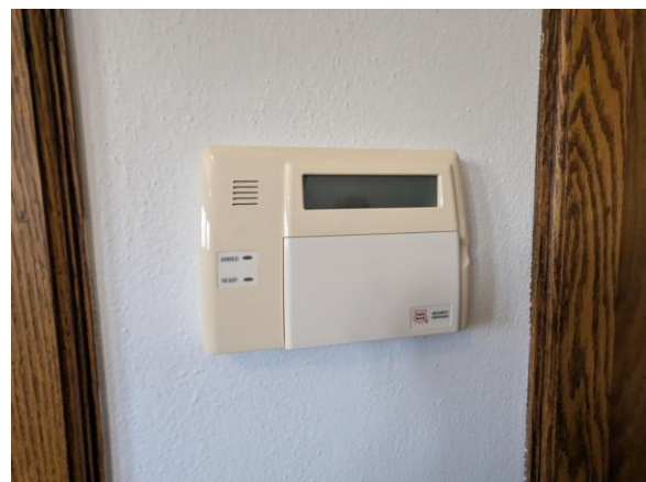
Figure 73 – Security System Keypad at Main Library Entrance (2026).
