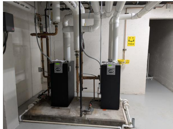
Figure 62 – New Hot Water Boiler Plant in Basement (2026).
