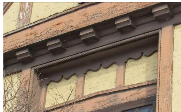
Figure 15 – The stucco and trim have exquisite detail, notice the rope mould and brackets (2026).
