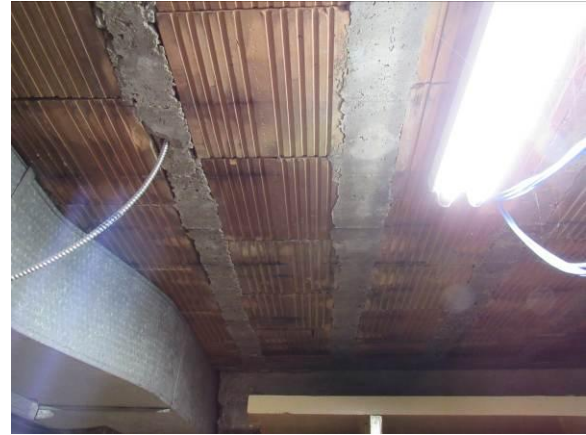
Figure 48 – Concrete floor joist system, notice how the electrical conduit was drilled through the joist, not the clay tile (2026).
