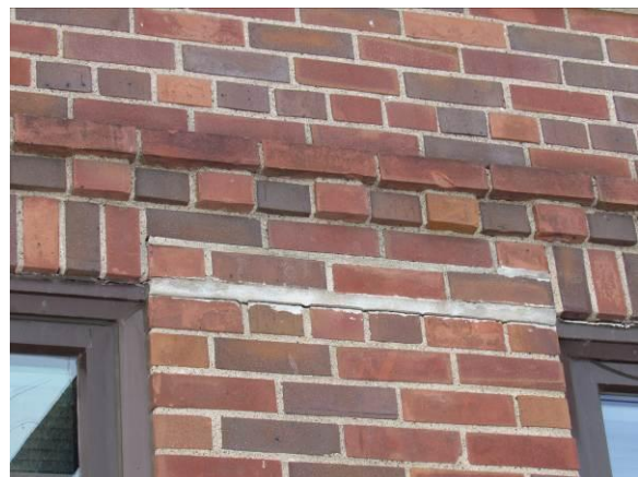
Figure 21 – Previous water infiltration may have rusted the steel lintel, pushing the bricks out of alignment(2026).
