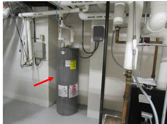
Figure 105 – The water heater is fairly new, circa 2024 (2026).
