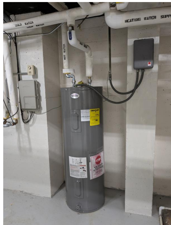
Figure 75 – Domestic Water Heater (2026).
