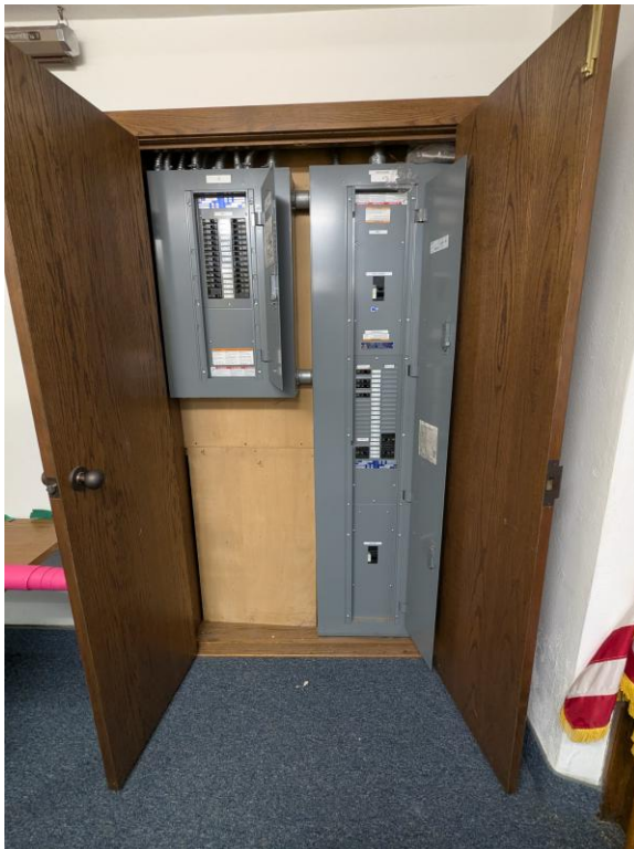
Figure 65 – New Electrical Service and Distribution Equipment (2026).
