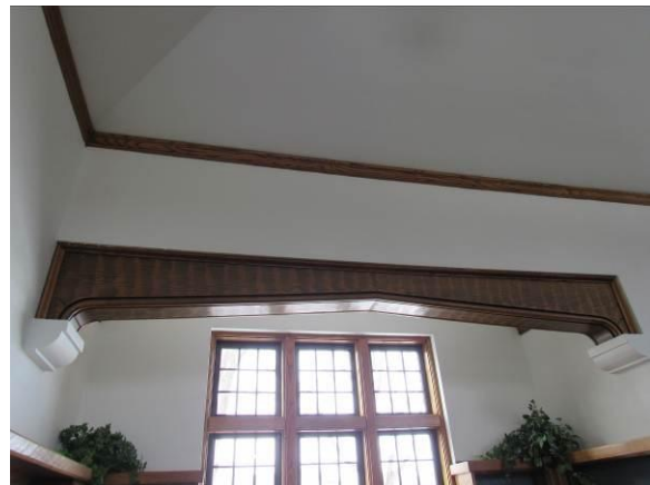
Figure 54 – The wood beams at the openings are decorative, the structure is above (2026).
