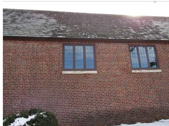
Figure 17 – The darker masonry near grade has been saturated with moisture (2026).
