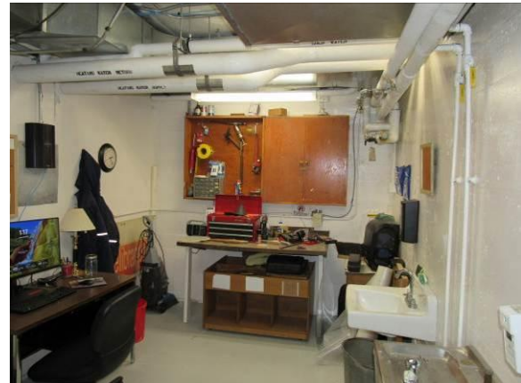
Figure 112 – The mechanical spaces are very clean and organized (2026).
