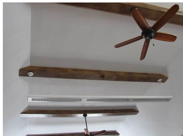
Figure 55 – The faux beams at the ceiling are decorative, not structural (2026).
