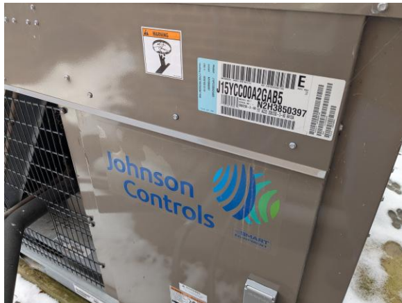
Figure 63 – New Air Conditioning Unit installed on Grade outside Building Entrance (2026).
