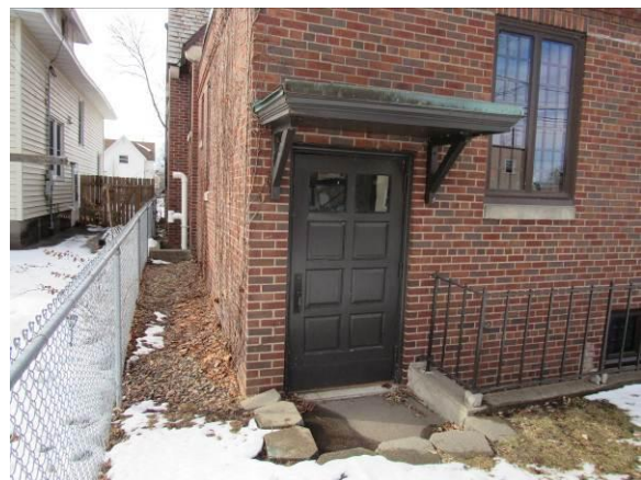
Figure 20 – Grade is above the threshold for the door leading to the basement (2026).
