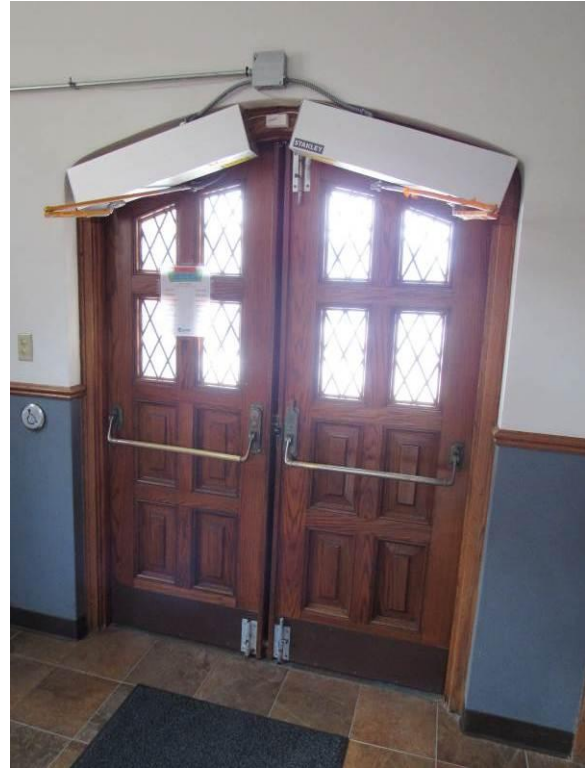
Figure 38 – The front doors have auto-operators to try and meet ADA req's (2026).
