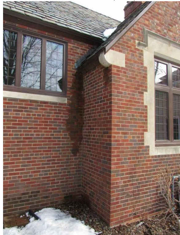
Figure 52 – The biggest threat to the masonry is water infiltration (2026).
