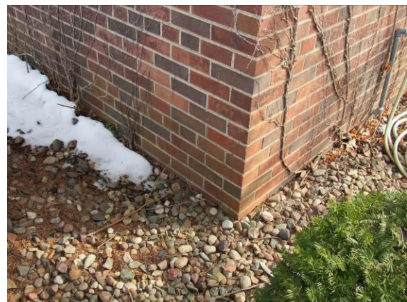
Figure 18 – The face brick runs below grade, notice the ivy (2026).
