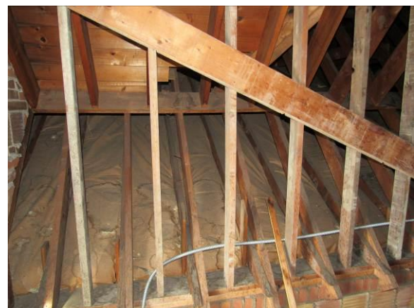
Figure 57 – The attic is a mixture of walls, rafters and collar ties all constructed with dimensional lumber (2026).
